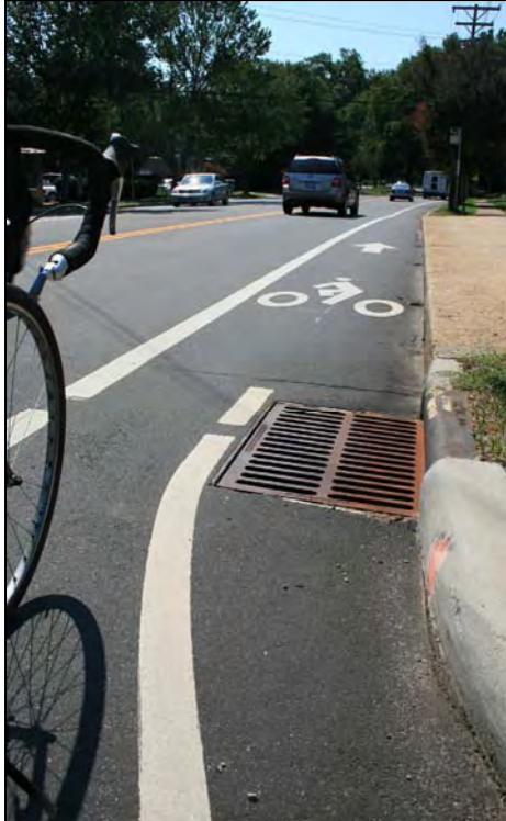
Dangerous grates, cracks, or holes should be fixed, while some hazards can be marked so that bicyclists can avoid them.
